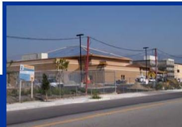
Citrus Continuation High School The official groundbreaking for the new facility was held on November 4, 2009. Construction is ongoing, the school will open in 2011.
